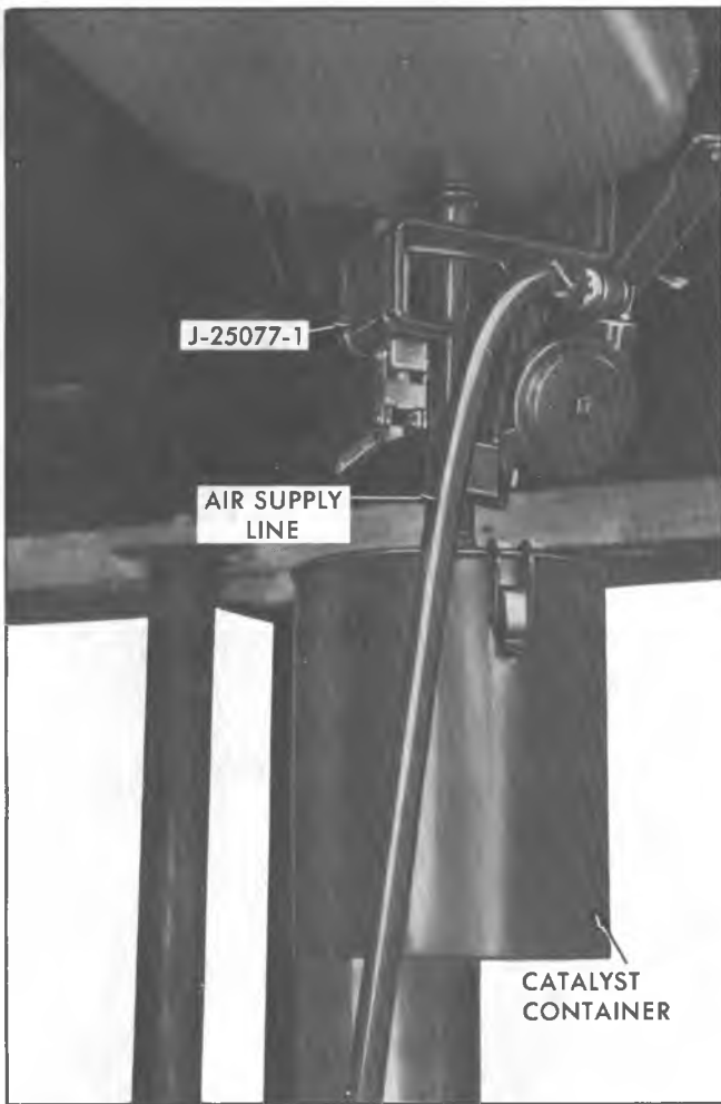
Fig. 8-Container Installed on Vibrator
